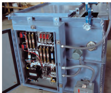
The inside of the switchgear box.
