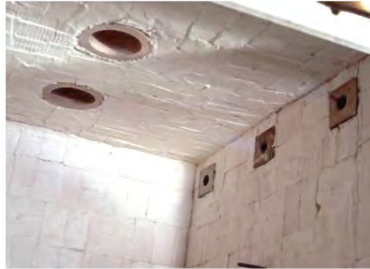
Burner blocks are along the top side; flues are at top.
