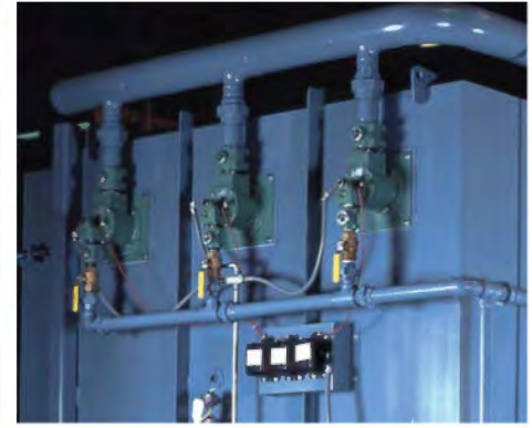
The gas and air train is all neatly hard piped.
