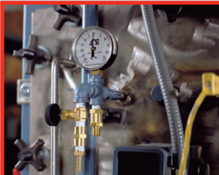
Retort pressure gauge & test bib
